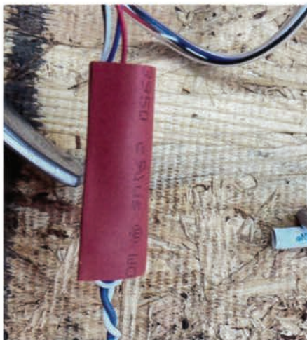
Figure 17. A piece of heat shrink tubing keeps everything neatly in place.
