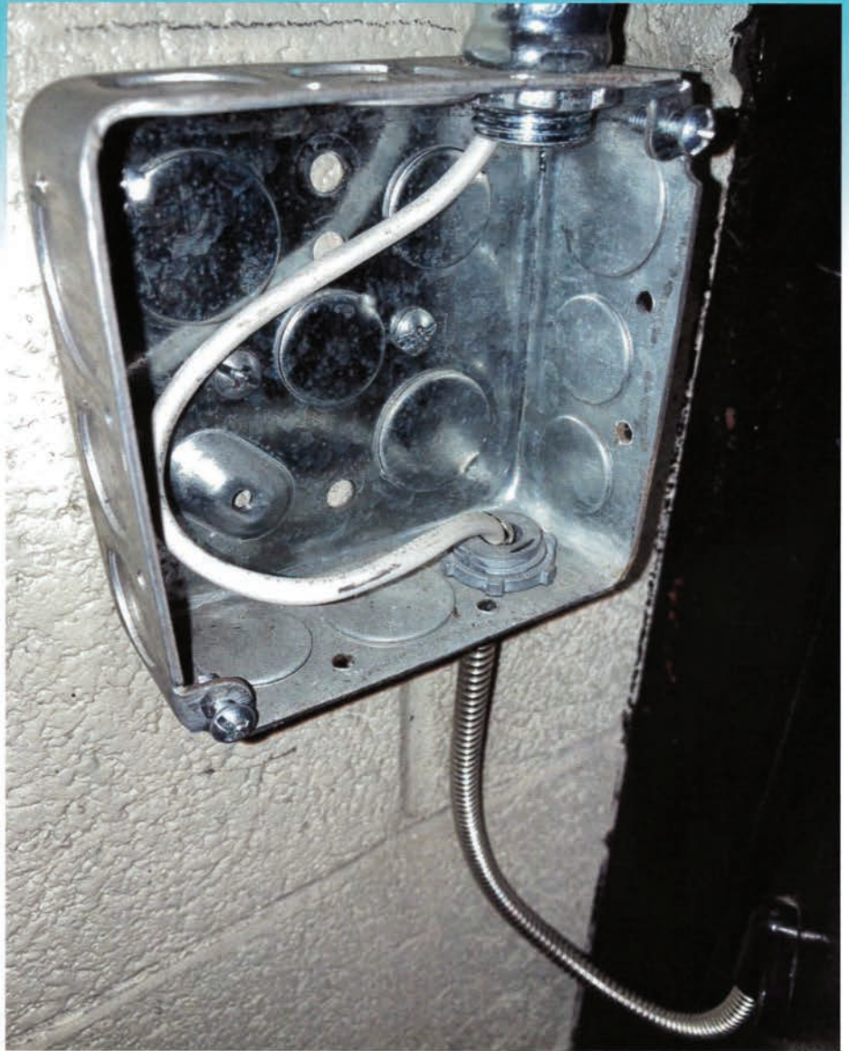
Figure 1. The electrical workbox was just used as a pass-through for the power wire.
