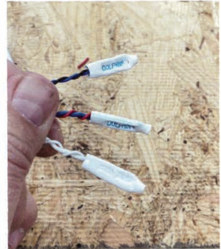
Figure 16. You can see the final connections.
