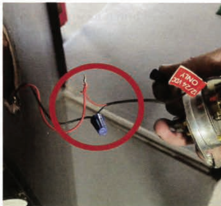
Figure 2. The power wires were attached to the lock with twist-on wire nuts.
