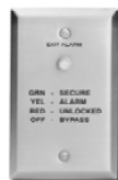
101-1A The single station annunciator is equipped with a tri-colored LED and audible alarm.
